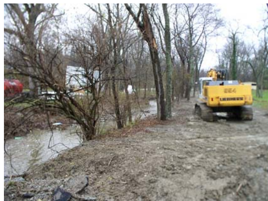
Lack of erosion controls near stream
