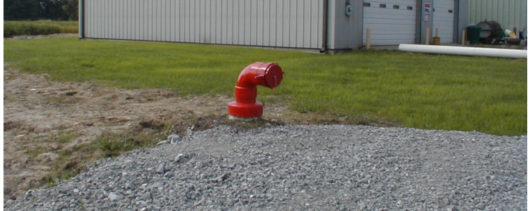
411s used as a topper for a heavy use area near a dry hydrant.
