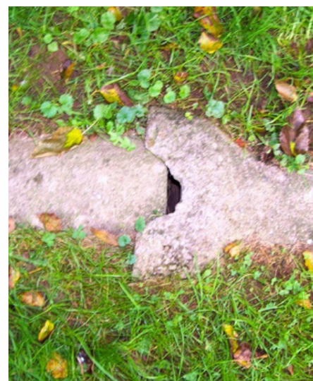
Failing concrete storm water pipe.
