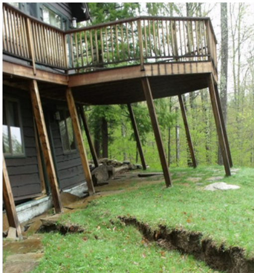
Land movement is occurring here, you can see the ground splitting.
