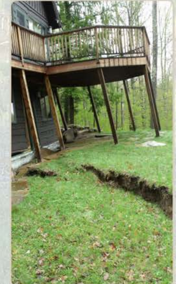
Land movement is occurring here, you can see the ground splitting.
